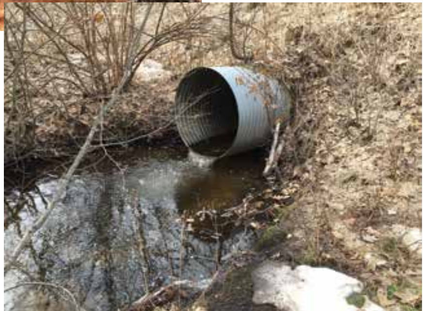
Perched culvert in Northern MI.
