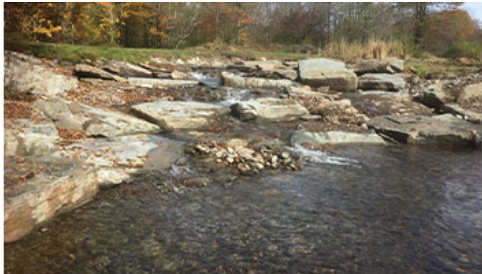
Frog Hollow, Tributary to Willowemoc Creek, after construction reconnecting 3 miles of spawning habitat.
