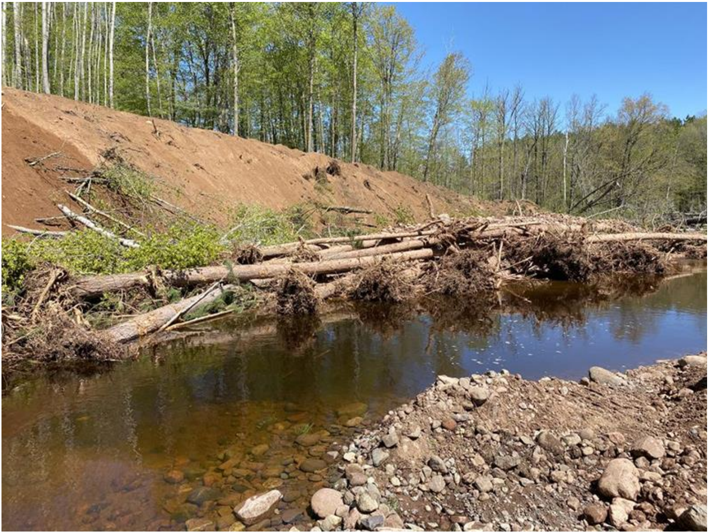
A 150-foot log jam built from trees harvested from the site helps prevent erosion and provides deep pool habitat and hiding cover for fish.
