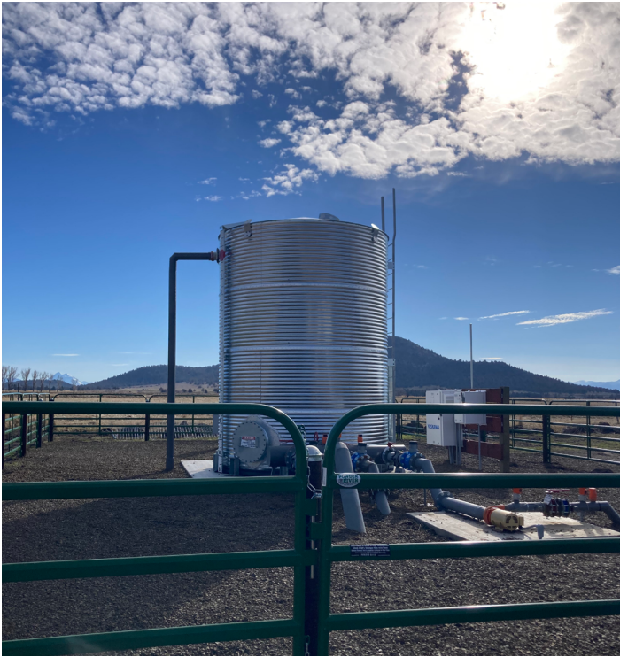
Figure 3. Main tank of new pressurized stockwater system which will allow for more efficient year-round livestock watering and will remove cattle from the stream
