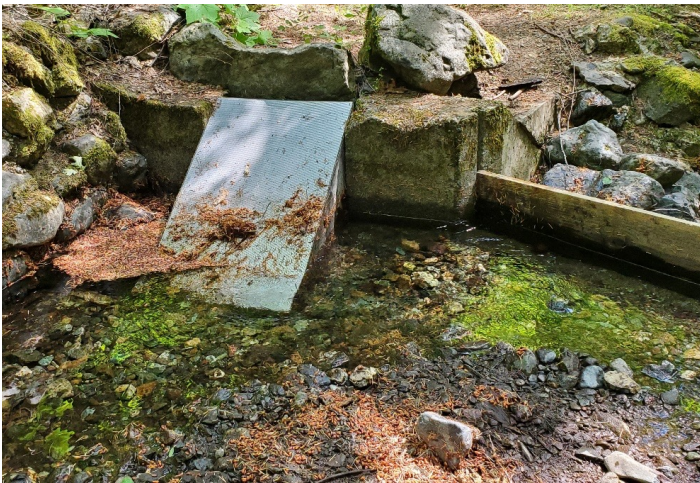
Figure 4. The current fish screen that will be replaced with a lower maintenance screen.
