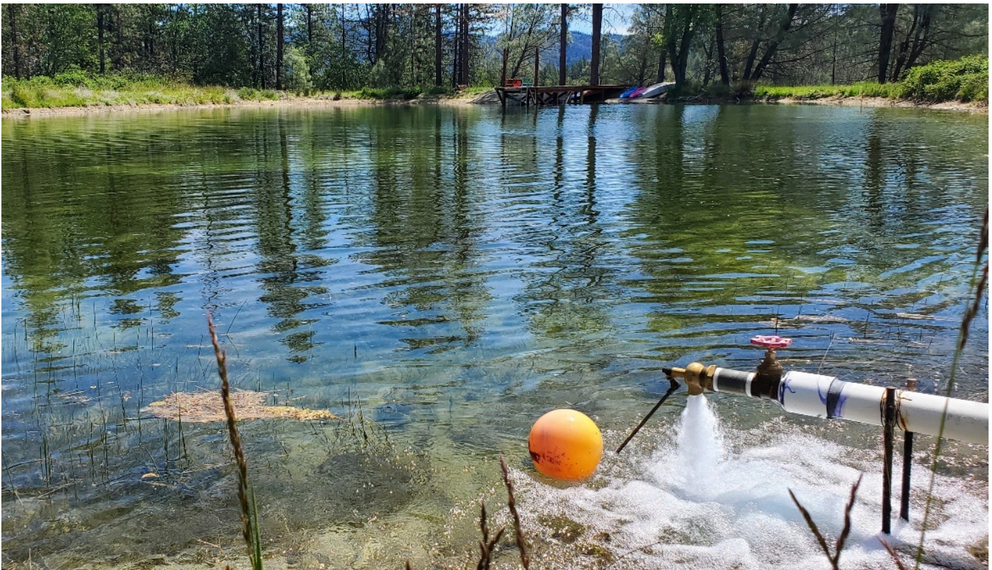
Figure 2. The trickle fill pond is being filled prior to the forbearance period. Note the orange ball attached to a float valve to stop the flow when the pond is full.
