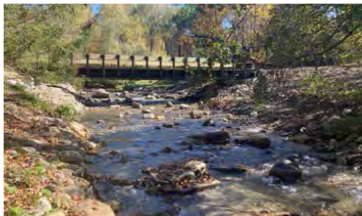
AFTER: Removal of the dam opened up 6 miles of previously inaccessible upstream coldwater habitat.
