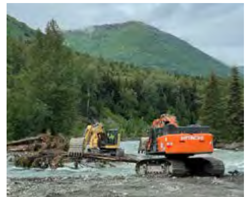
Construction of a new stream channel in Resurrection Creek, 2023, outside Hope, Alaska.
