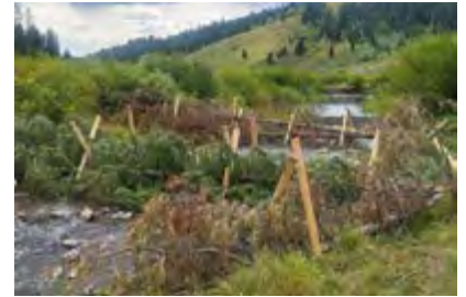
Post-assisted log structures installed as part of a PBR project on North Fork Tincup Creek, Idaho.
