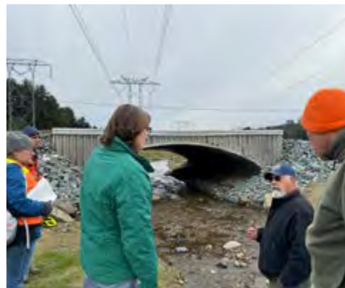
New Hampshire Stream Restoration Specialist with agency and municipal partners at the Childs Brook culvert replacement project in Bath, New Hampshire.
