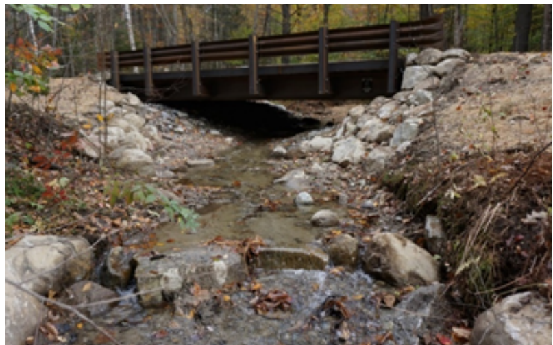
A new bridge was installed over Ryan Brook under Perch Pond Road in Campton, New Hampshire
