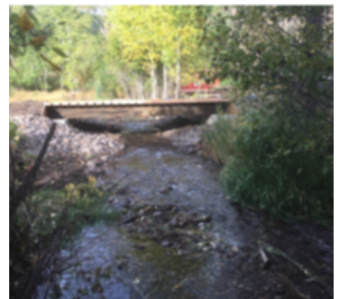
The top photo is the old culvert. The bottom photo is of the new bridge on Brewster Creek, Rock creek drainage, MT.
