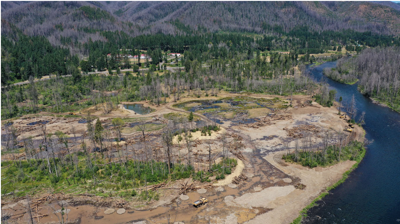
Figure 15—Hauling wood and moving sediment along the McKenzie River floodplain valley-bottom reset project at Finn Rock reach, Willamette National Forest, OR in 2022. Courtesy photo by McKenzie River Trust/Steve Smith Photography.
