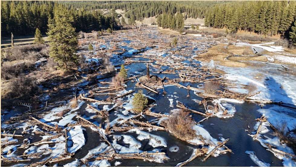
Figure 6—Camp Creek Reach 1 valley bottom restoration the winter following large wood additions and valley bottom restoration that used wood derived from a large vegetation management project where commercial, non-commercial, fuels, and forest health treatments were completed. Malheur National Forest, OR in 2024. Forest Service photo.
